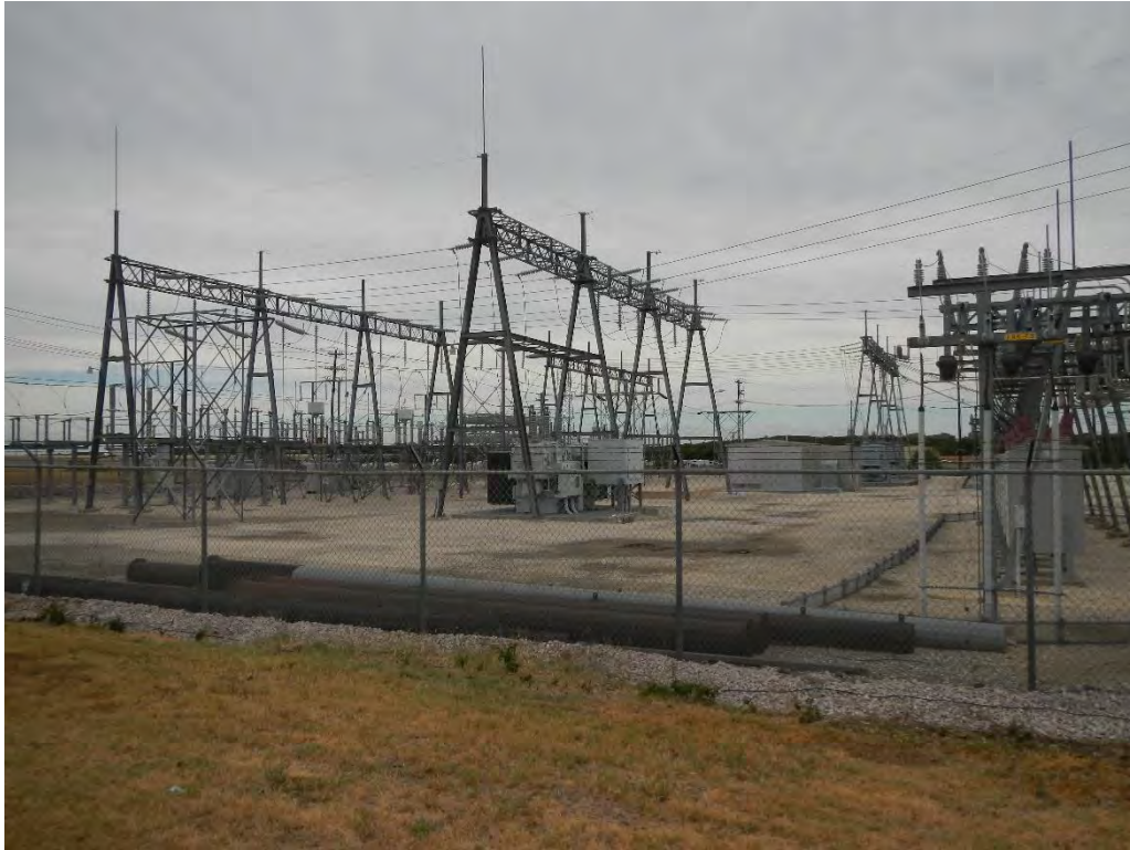
Photo 11: Electrical substation located on the southwest corner of Hero Way and 183A, facing southeast.
